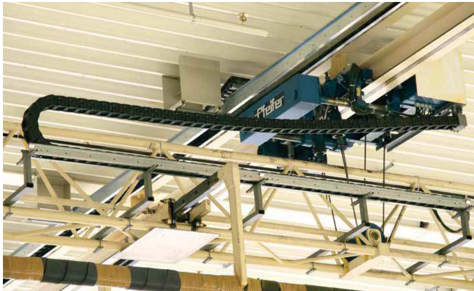
Handling unit indoor crane - long unsupported span with an igus® E4 series
